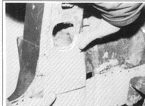
Figure 6. Repair plate and curved recess.
